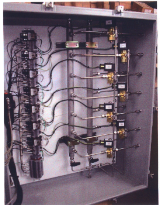
Control Panel for Air-Actuated Diaphragm Valves (Interior View)
