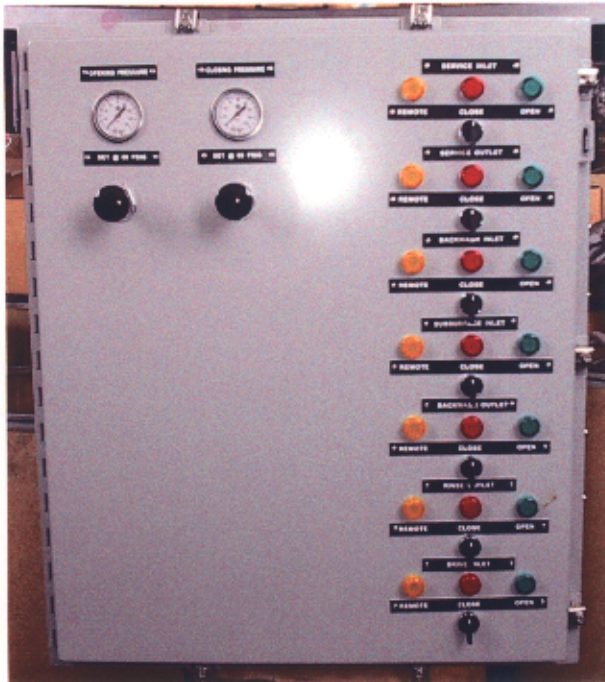
Control Panel for Air-Actuated Diaphragm Valves
